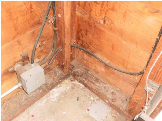
There is electrical circuit wiring that is not considered adequately protected in the detached garage at the west wall.
