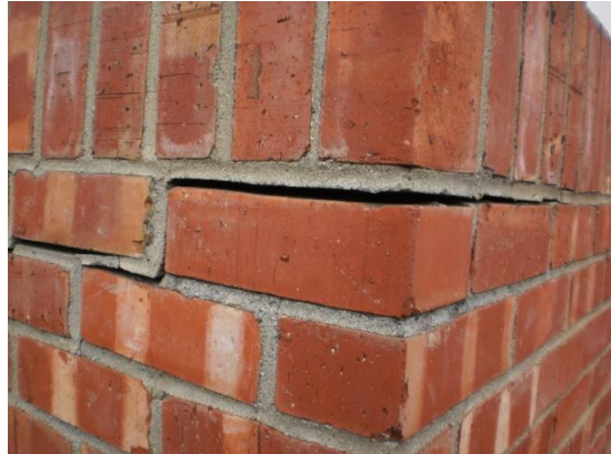
There is evidence of large cracks at the top of the chimney.
