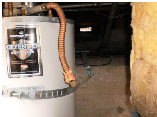
The discharge piping for the temperature/pressure relief valve terminates in the basement.
