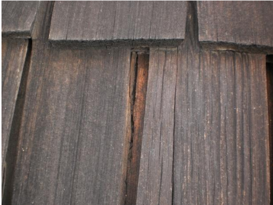
There is exposed underlayment at the south side of the house.
