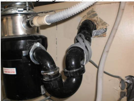
The drainage piping in the cabinet below the kitchen sink is an improper design.
