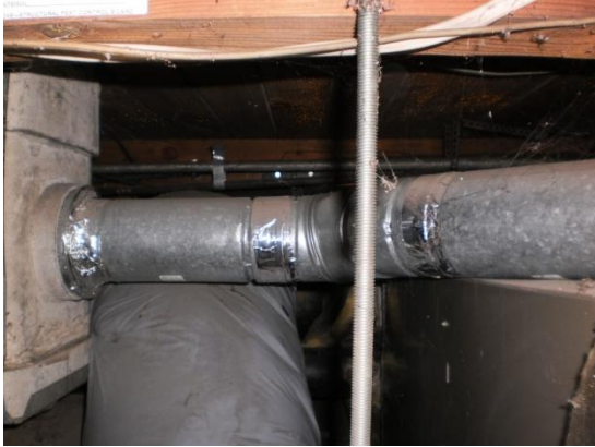
The flue serving the heating unit is improperly sloped in the basement.
